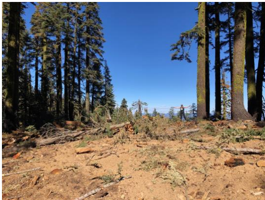
Dozerline built over the Pacific Crest Trail in the Bucks Lake Wilderness Area during the 2021 Dixie Fire. Photo Credit: Darrel Jury
